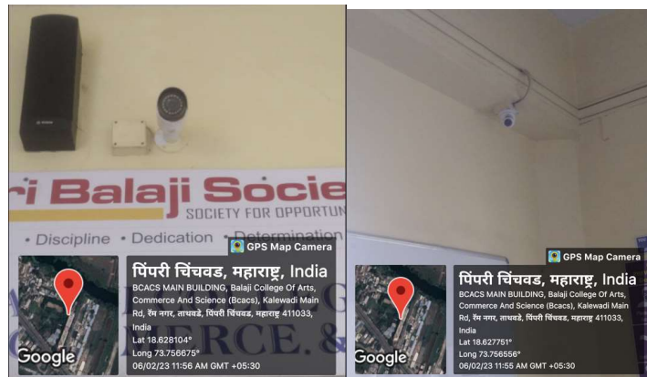
Some of the CCTV Cameras installed in BCACS
